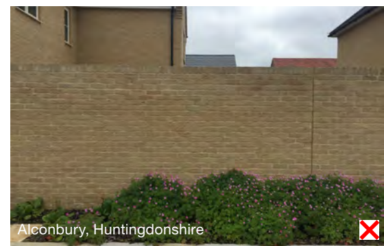
Figure 5.44: Side boundaries with a blank wall as not sufficient greenery was planted
