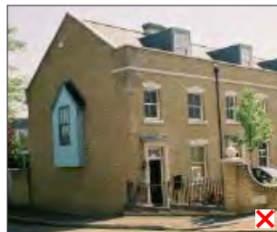
Figure 5.25 - Poor example of a retroactively incorporated window on a gable end of a terrace
