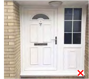
Figure 5.51: No uPVC doors permitted on primary entrances
