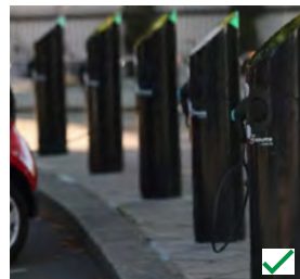
Figure 5.84: Electric car charging points
